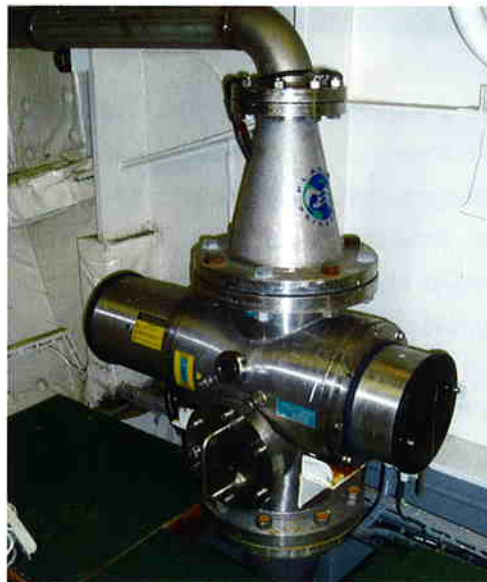
MBR permeate disinfection system
